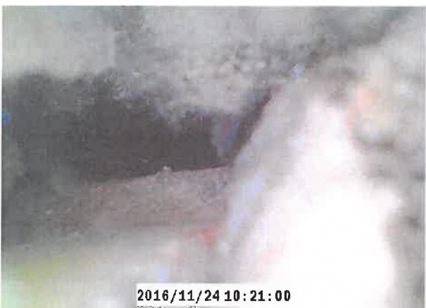
2016/11/24 10:21:00 Voids within cavity
