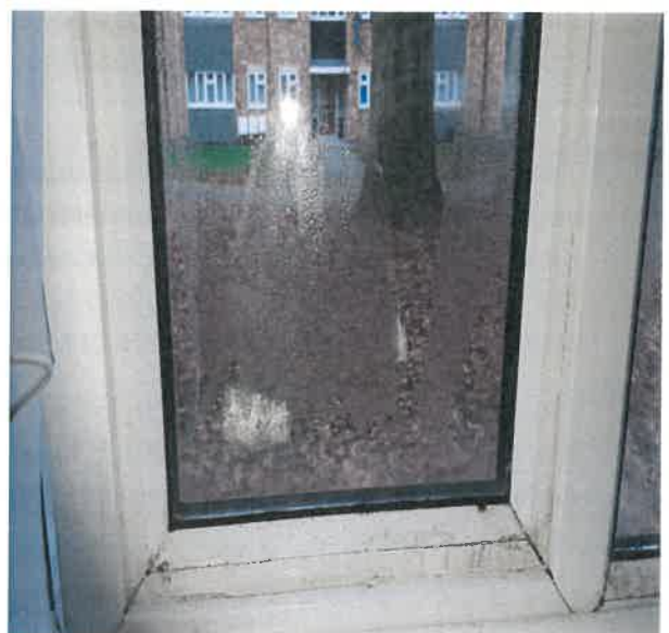
Excessive condensation on cold spots
