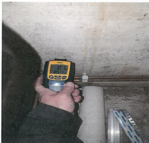
Accelerated mould growth high moisture
