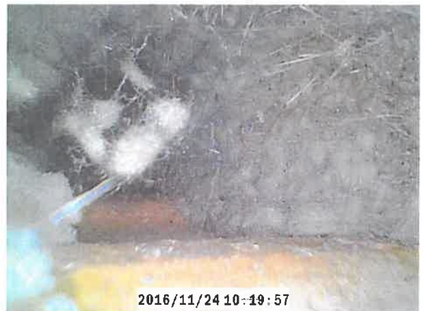
2016/11/24 10:19:57 Voids within cavity causing cold spots
