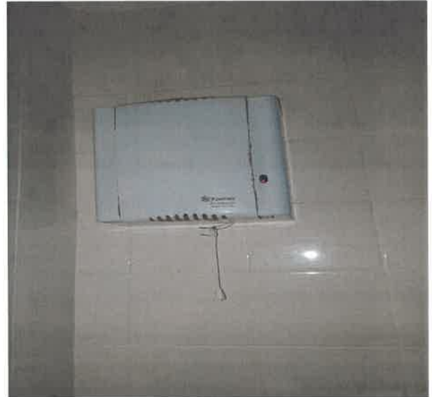
inadequate ventilation for building
