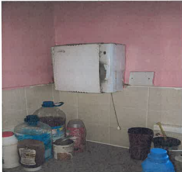
Poorly sited, poorly maintained
