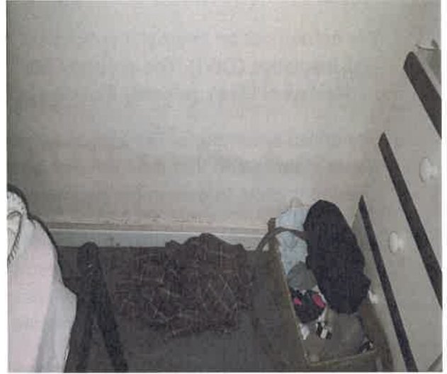
Moisture penetration of internal wall
