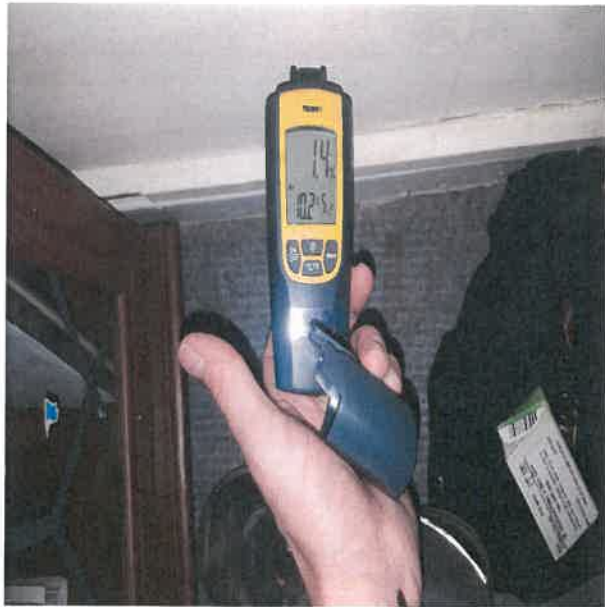
High moisture content of internal walls
