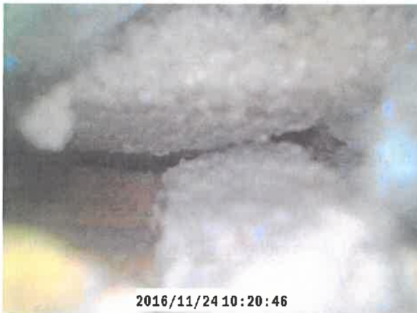
2016/11/24 10:20:46 Debris within cavity causing obstruction
