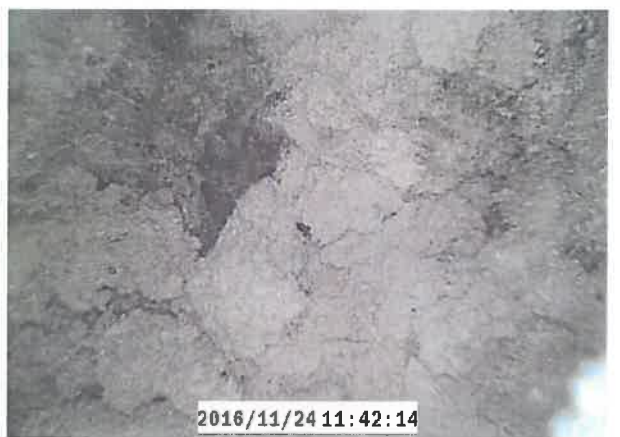
2016/11/24 11:42:14 Debris within cavity
